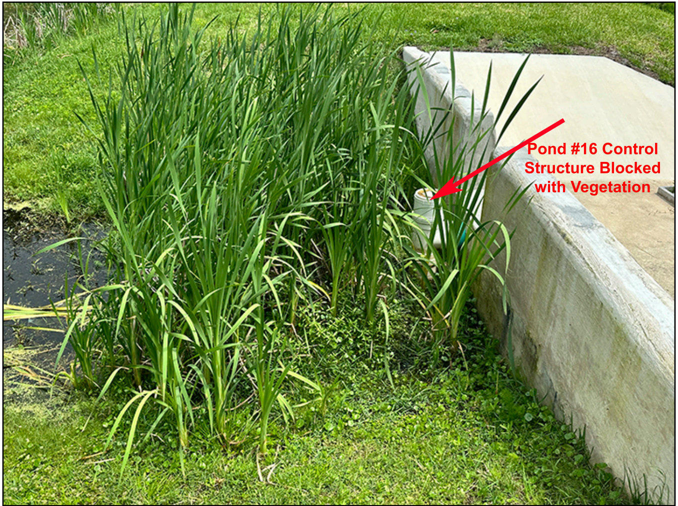
Figure No. 7 - Pond #16 control structure blocked by aquatic vegetation.
